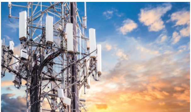
5G Transmission Towers
